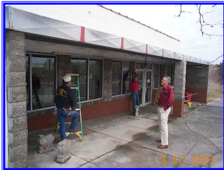
New Alternative High School Storefront Thermal glass, insulated walls, improved structure Architectural design fits School District model. State in-house design and project management. Project Bid 10% below design estimate - no change orders!
