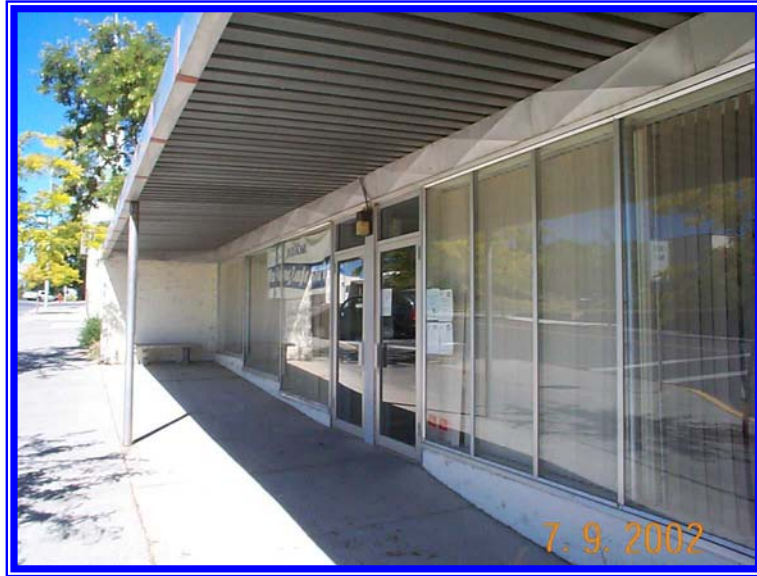
Original Alternative High School Storefront. Single-pane, leaking, no insulation.
