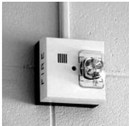
Morehead State University installed fire alarms in each dorm room after a student was killed in a fire at Murray State University in Kentucky in 1998.
