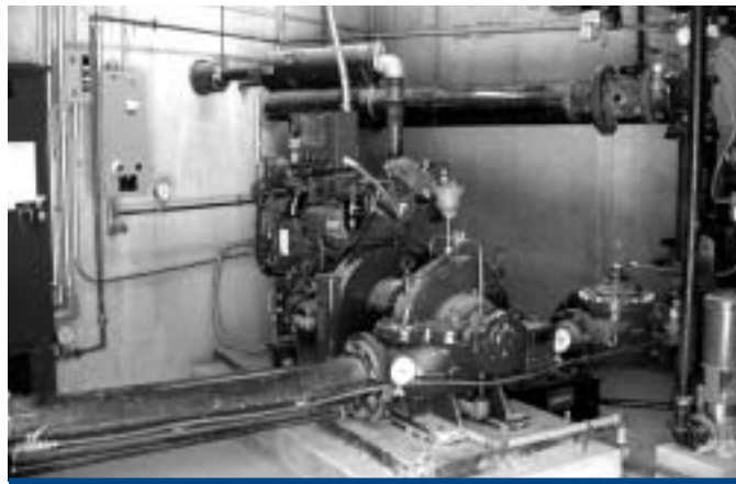
Morehead State University in Morehead, Ky., is installing pumps to increase water pressure at high-rise dorms.
